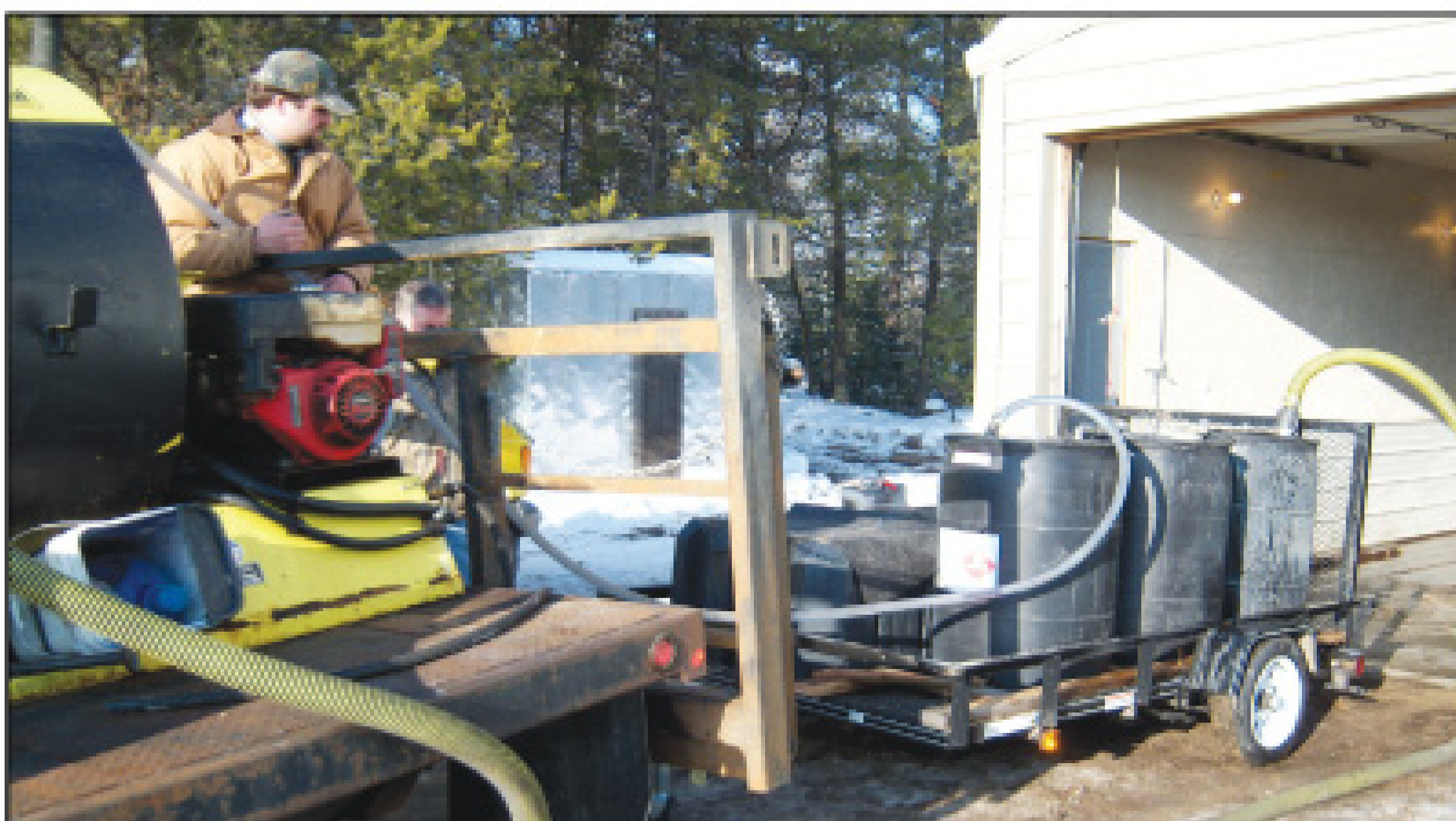
Technician Jeremiah McMillan loads water on a vacuum truck, using a mix of 10- to 30-percent methanol and 2 pounds of salt per gallon to avoid freezing.
