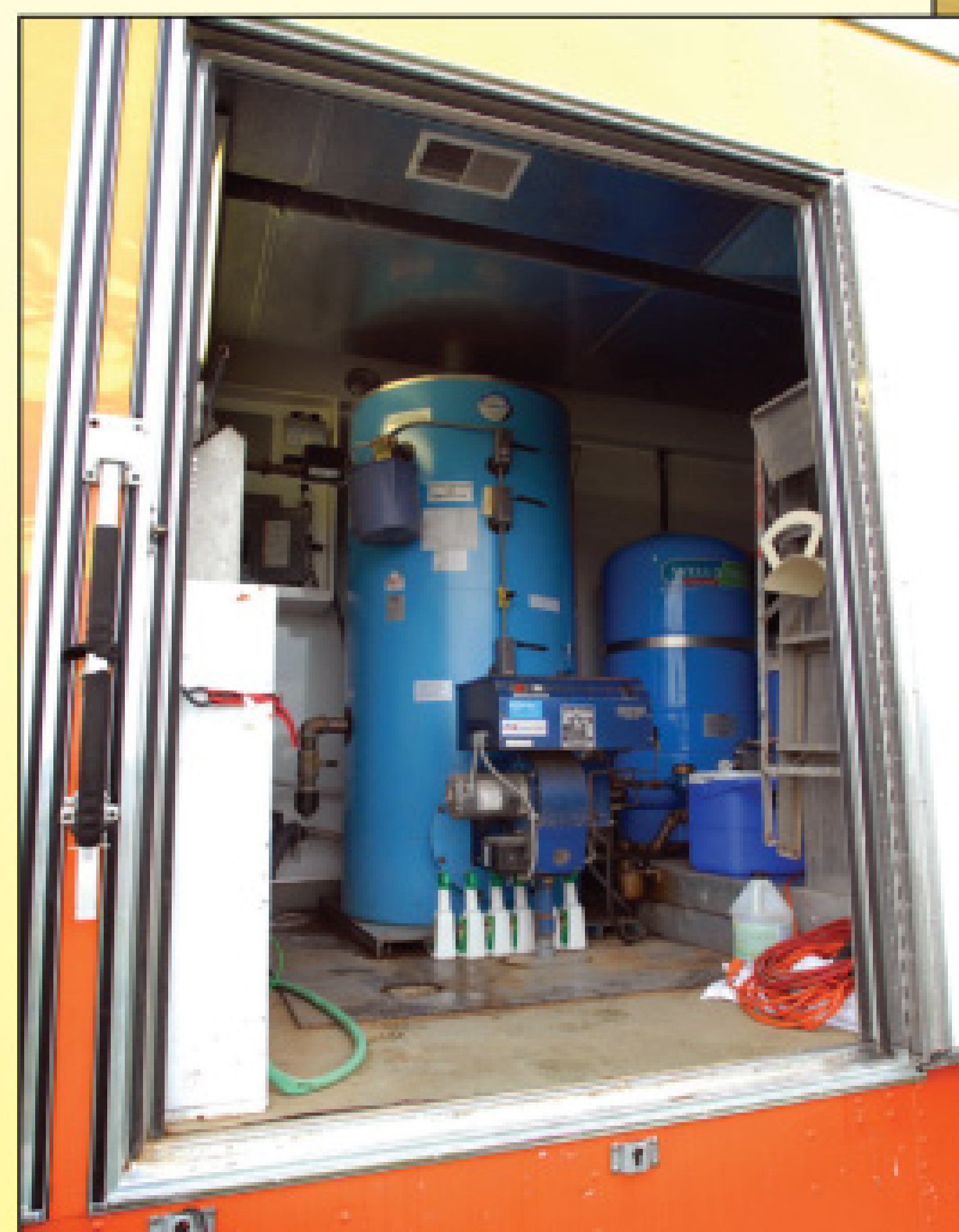
Below, the diesel-powered water heater is housed at the front of the shower trailer.
