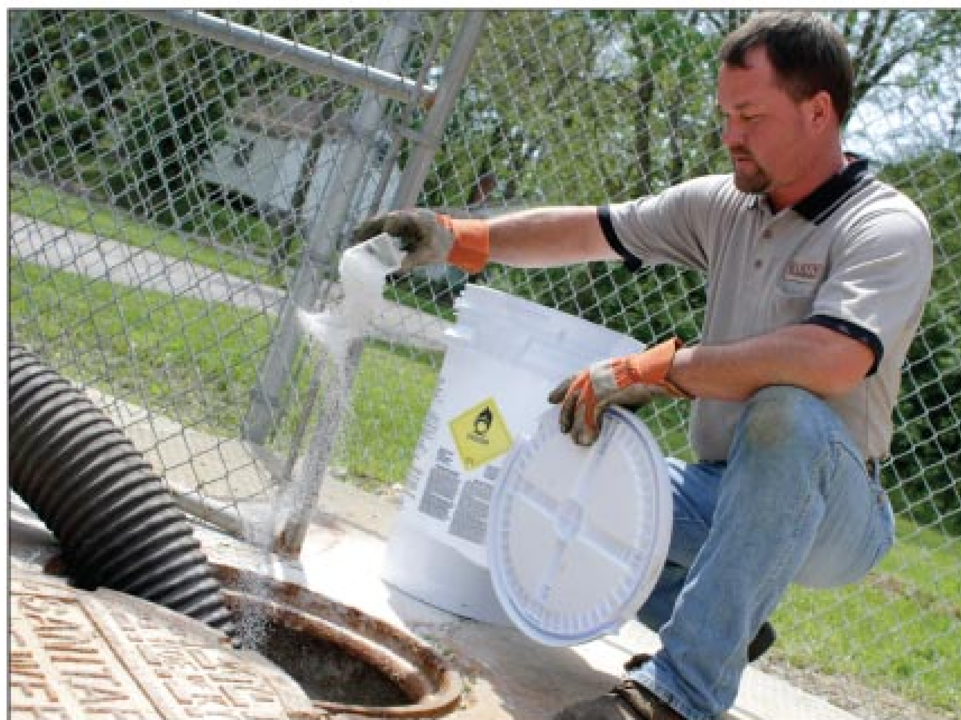
Technician Casey Jones pours a chlorine product into a tank at the Paris, Tenn., treatment plant to keep odors down.
