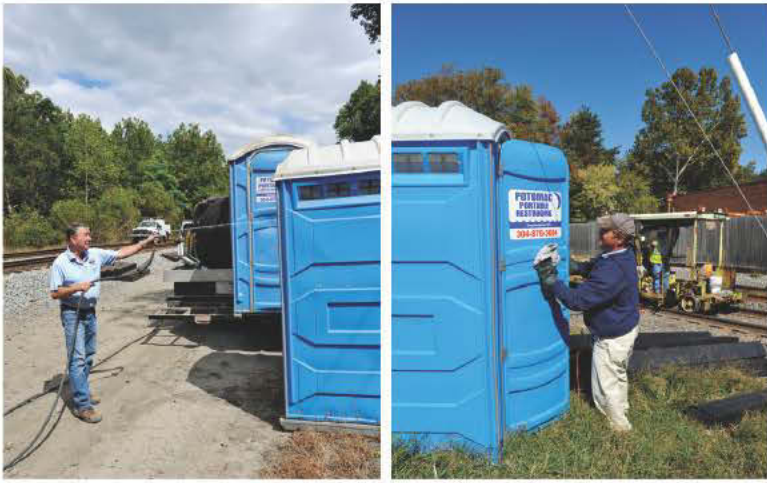
Above: (Left) Fighting dusty conditions, Jack Meyer powerwashes a restroom as a maintenance crew drives a truck down the railroad tracks. (Right) Technician Scott Hill wipes dust from a restroom delivered ahead of the work crews. In the background, a CSX crew marks railroad ties to be replaced.
