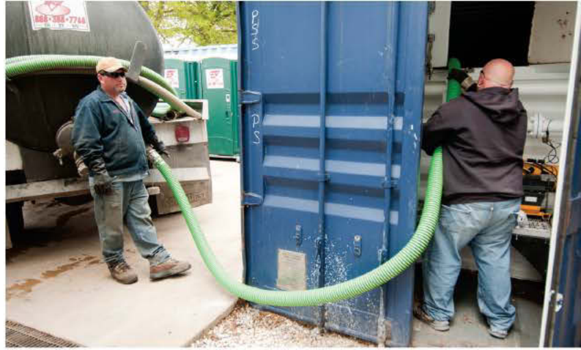
Terry Summers (left) and Wes Hackworth pump a 10,000-gallon waste processing station built by JOTS.
