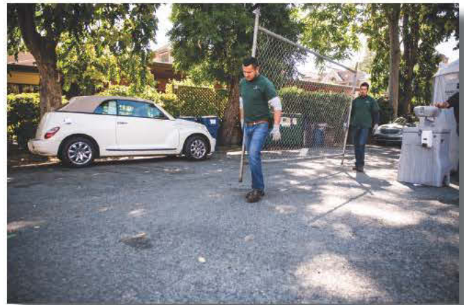
Tearing down at a site services location, Juan Mayoral and Guillermo Molina remove fencing in Danville, Calif. vvv
