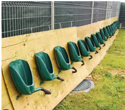
Right: KM secured Satellite urinal units to plywood sheets and plumbed into a pair of Fralo (Roth Global) tanks in a common men's portable sanitation area.
