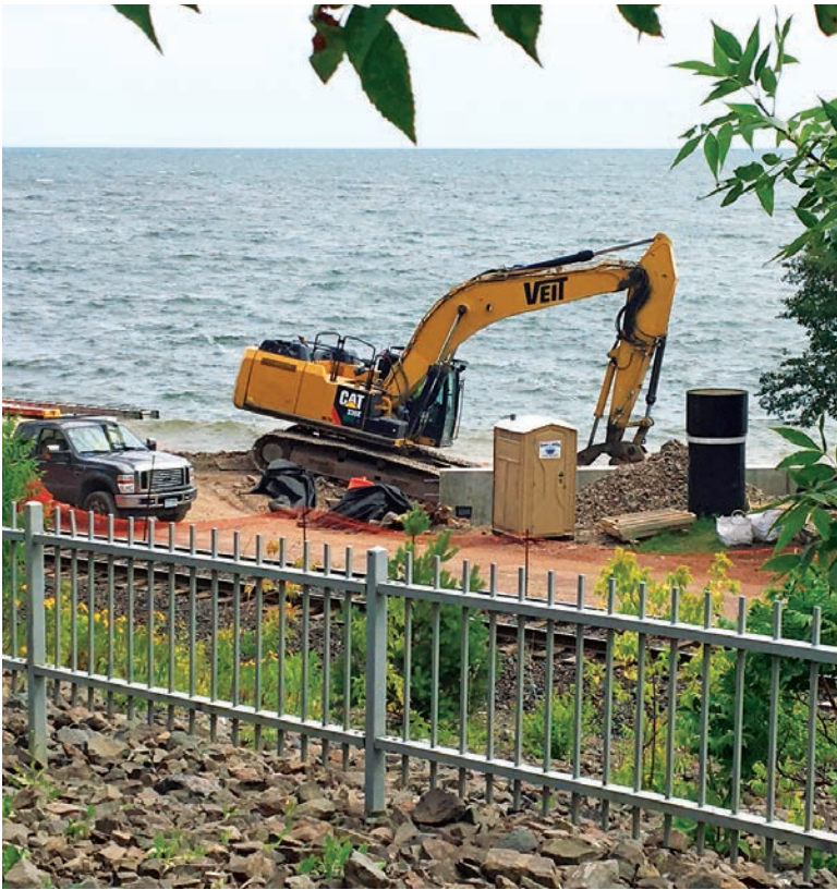
Above: There is nothing to object to in this restroom placement at a construction site along a Lake Superior waterfront trail.
