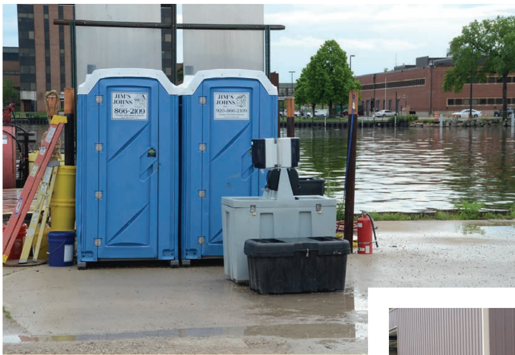
Right: A typical riverside construction site setup in Green Bay features restrooms from Satellite Industries and a T.S.F. Company hand-wash station.
