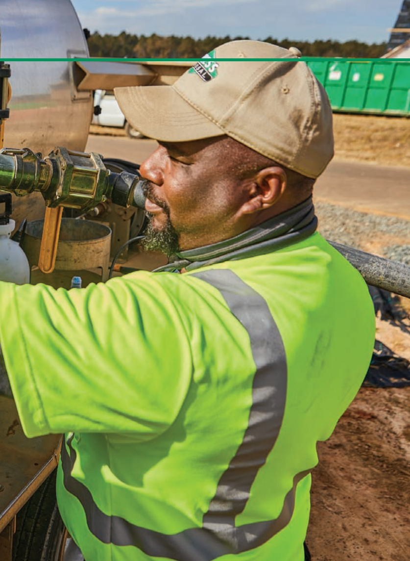
Left: Technician Oneal Barge returns the suction hose to his truck, built out by FlowMark and carrying a National Vacuum Equipment pump.
