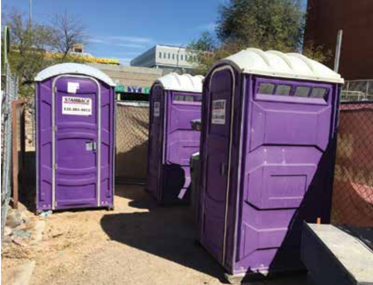
These PolyJohn restrooms are placed at a construction site at the University of Arizona in Tucson, Arizona. In regulatory changes, Canadian officials would like to require a women-only restroom on every construction site. (Photo by Jim Kneiszel)
