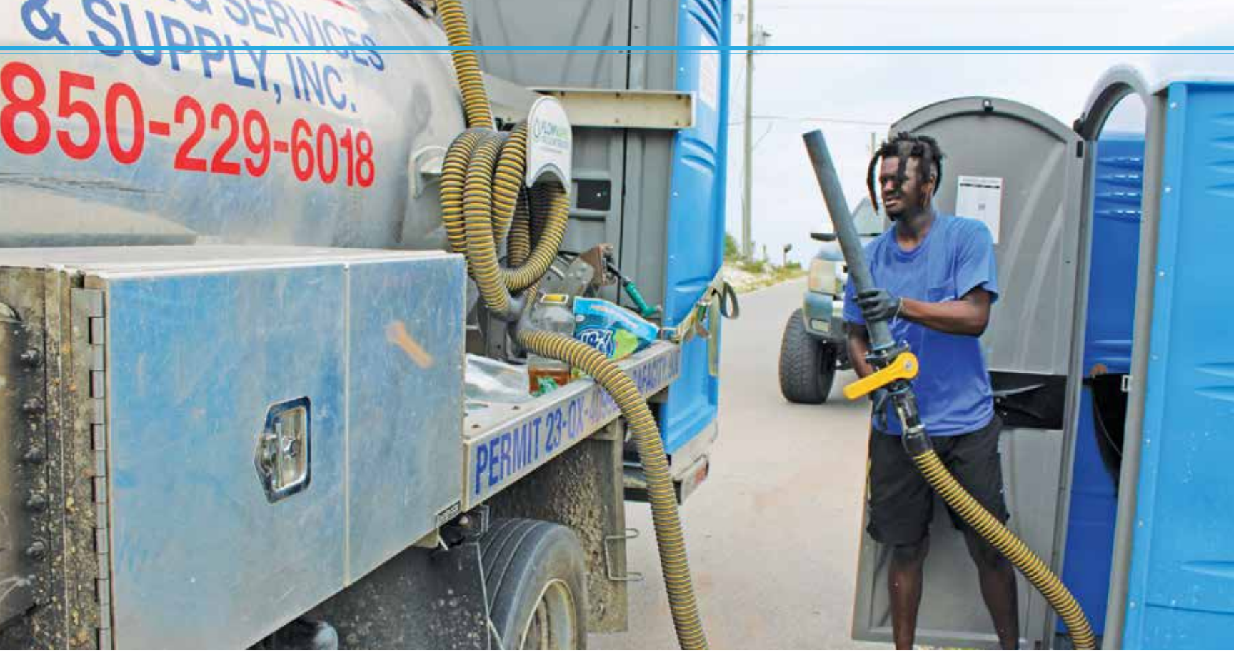
Above: Technician Neshon Gadson prepares to service an Armal restroom on his daily service route. The truck from FlowMark carrying a Bruder tank and Masport pump.
