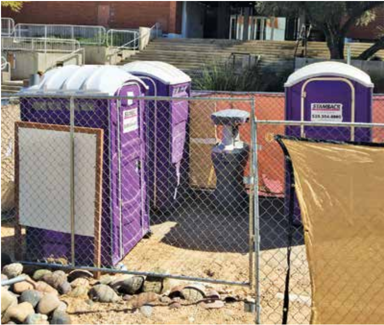
Above: Wire mesh temporary fencing is employed to secure PolyJohn restrooms and a hand-wash station at a University of Arizona construction site in Tucson, Arizona. (Photo by Jim Kneiszel)
