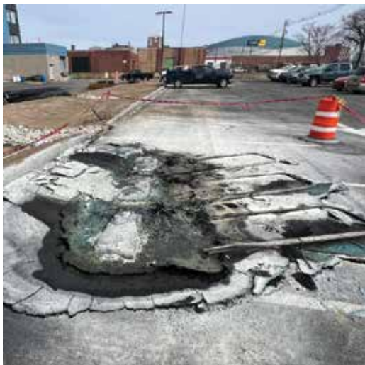
Arson left these three restrooms as a pile of melted plastic.
